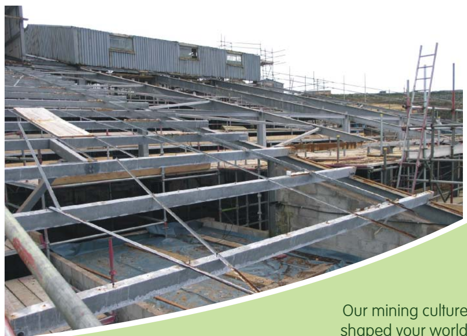
The roof of the mill building with the original sheet covering removed
