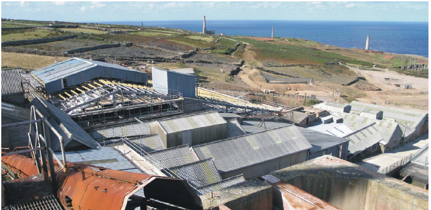
Years of exposure to the Atlantic wind and rain had taken its toll on the mill roof
