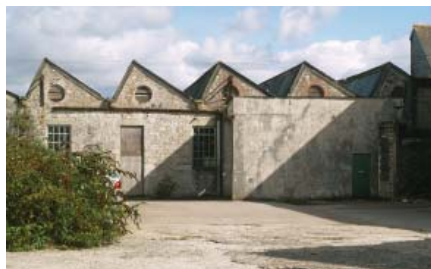
Early twentieth-century 'saw-tooth' roofline surmounting mid nineteenth-century wall of the earlier Burgess Foundry
