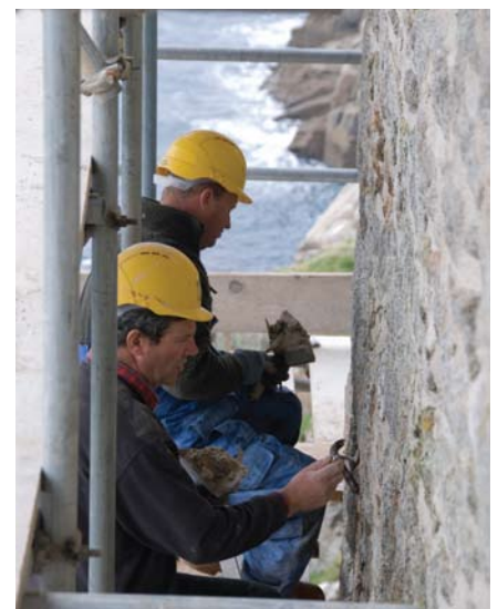
Above - working on the New Shaft engine house - Roger MacLean (rear) and Steve Flinders carefully re-point the walls using traditional techniques and lime based mortar.
