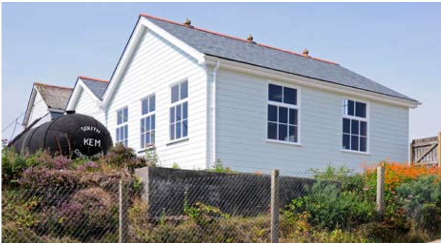
(Left) The rebuilt winder and compressor houses at King Edward Mine, Troon, now complete
