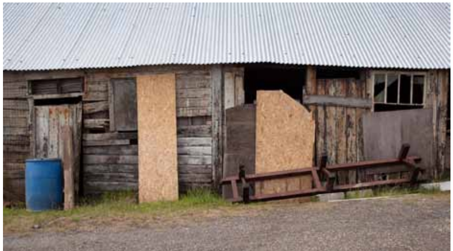
In need of attention, the timber-clad Assay House is part of the Grade II* Listed mine complex
