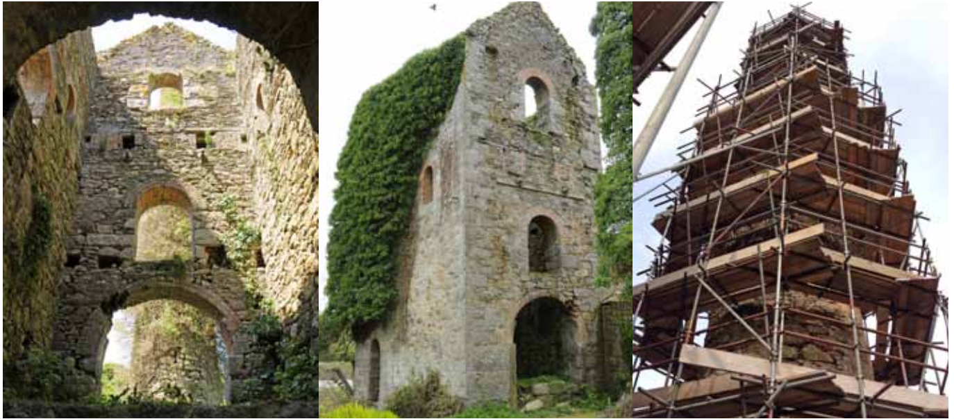
Above: The imposing pumping engine house and chimney (1856) at Wheal Busy, about to be conserved using Natural England Higher Level Stewardship funding
