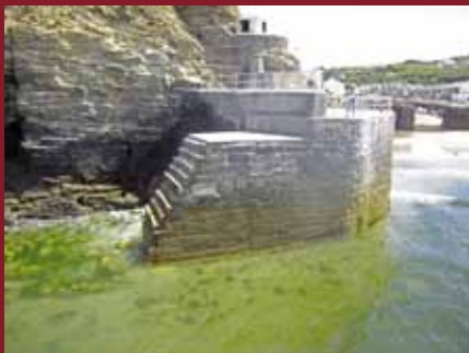
The northern extent of the Eastern Breakwater (above) which has been rebuilt using the original granite dimension-stone following extensive winter storm damage (main) (A. Brigden)
