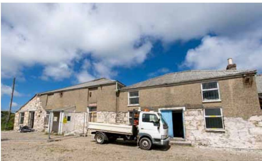
From left to right, the Mess Room, Count House and Smithy buildings, to be renovated as part of the current £2million workspace development project
