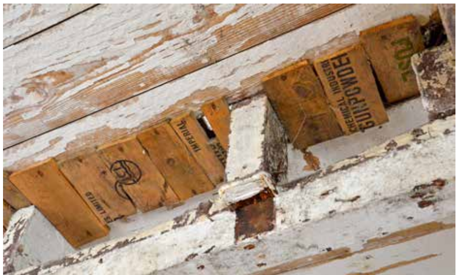
The Miners' Dry (the wash and change house), while in use (top) and during renovation. The cylindrical Cornish boiler provided both heating and hot water. The ceiling has been patched in former times using the timber slats from old packing cases of ICI safety fuse
