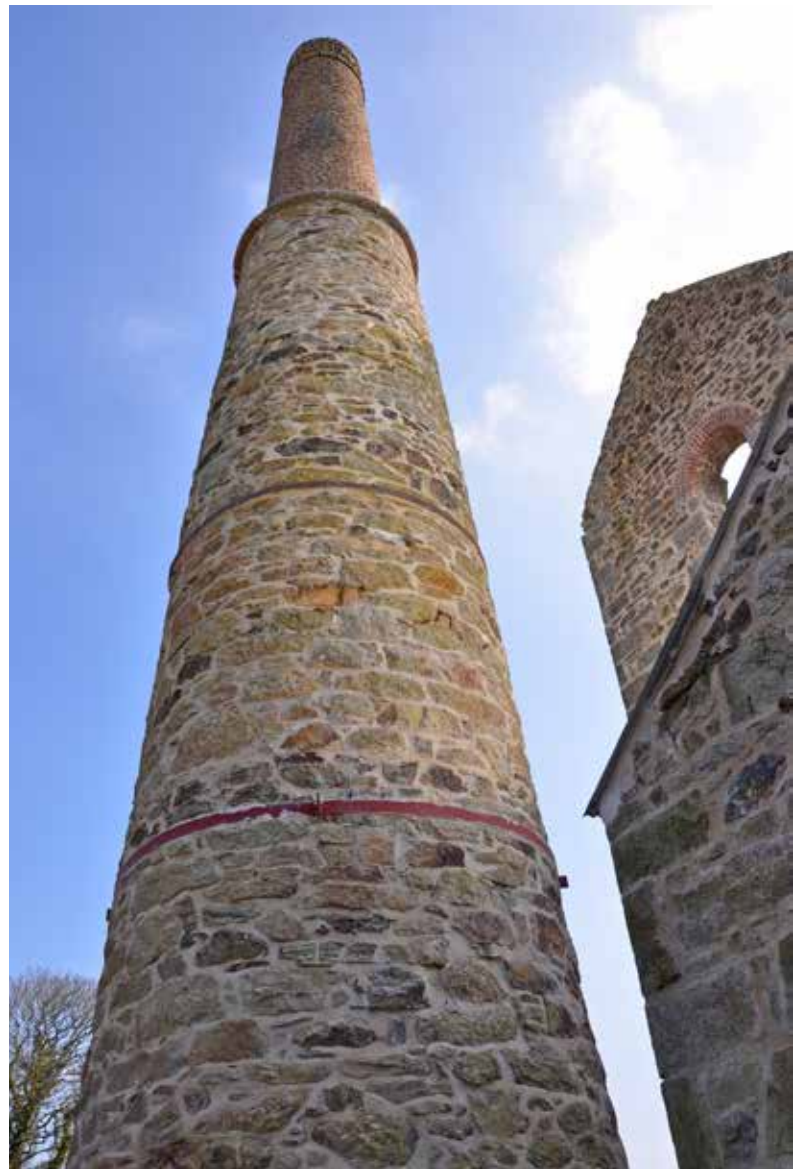
The restored chimney after repointing and the resetting of the uppermost brick courses
