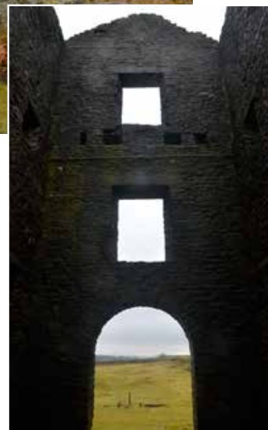
The interior of the pumping engine house at Magpie – testimony to the impact of the Cornish in the winning of lead
