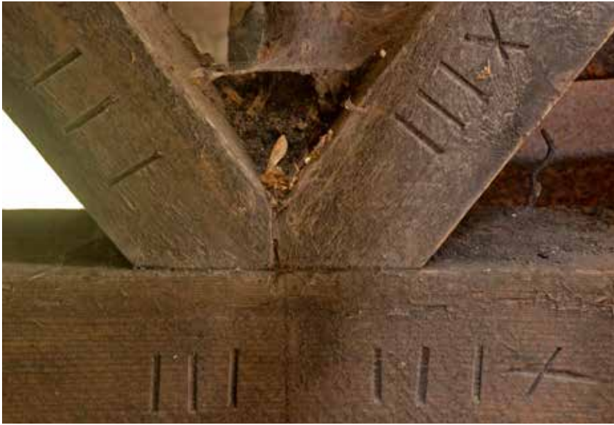
Carpenters' marks on roof trusses dating from the construction of the boiler house c.1909
