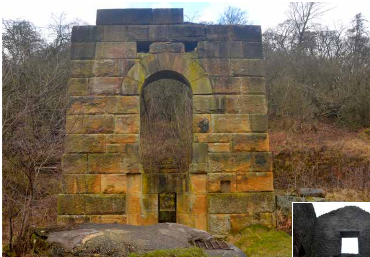
The bob wall at Millclose Mine, all that survives of the Cornish engine house here
