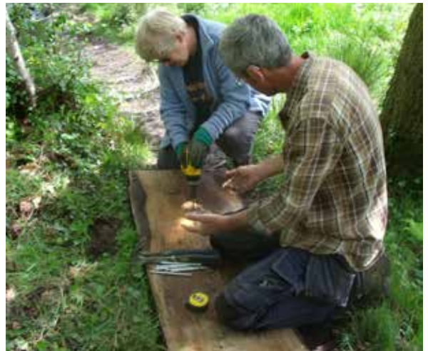
Volunteer co-ordinator Dave Readman gives a guiding hand to a volunteer replacing a bench at Okel Tor Mine
