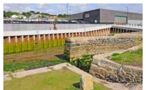
Views of the sluice gates at Carnsew Pool before and after reinstatement, with the sluice training wall at Carnsew Dock below
