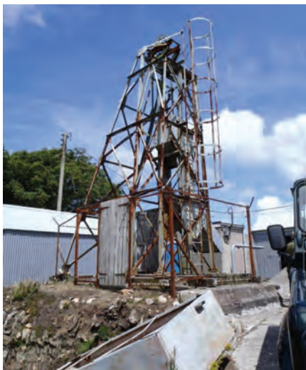
Below: the deteriorated headframe before restoration
