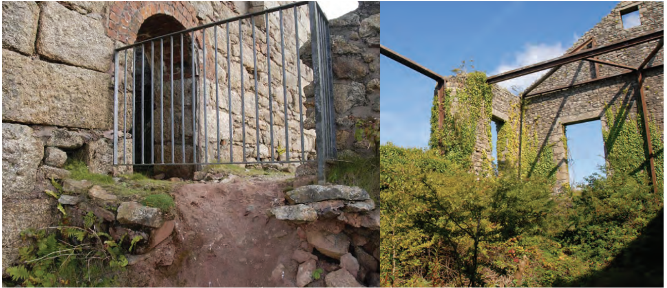
Above: problems with surface erosion at the West Basset Stamps site
