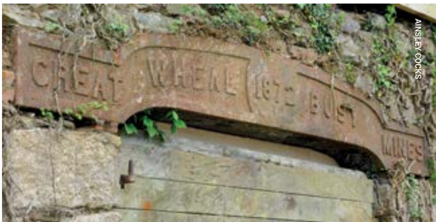
Above: One of the two impressive cast iron door lintels of the Smithy, manufactured by Perran Foundry in 1872.
